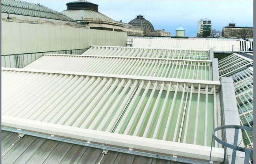
Tate Britain, London. Controllable Solarfin fins installed on top of Colt Azur rooflight systems.
