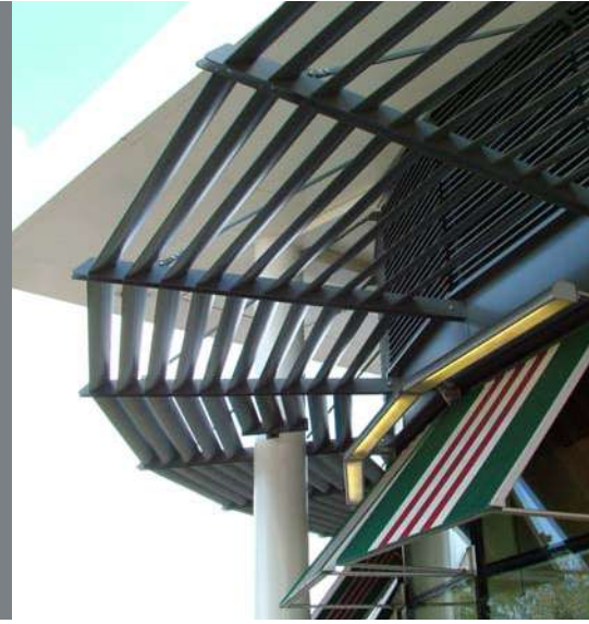
Castlepoint Shopping Centre, Bournemouth. Solarfin louvres set onto prefabricated faceted structure.
