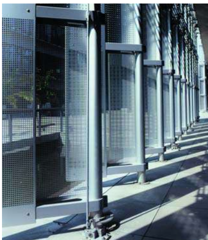
UTZ Offices, Berlin, Germany. Bespoke vertical solar shading fins that can be manually altered to control internal daylight levels.
