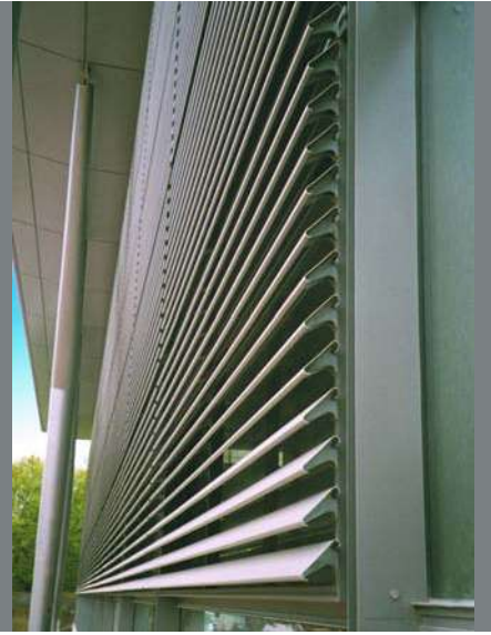
Clissold Leisure Centre, London. Vertical Solar C covers the glazing, which can be pivoted at an angle to facilitate easy cleaning of the glass behind.
